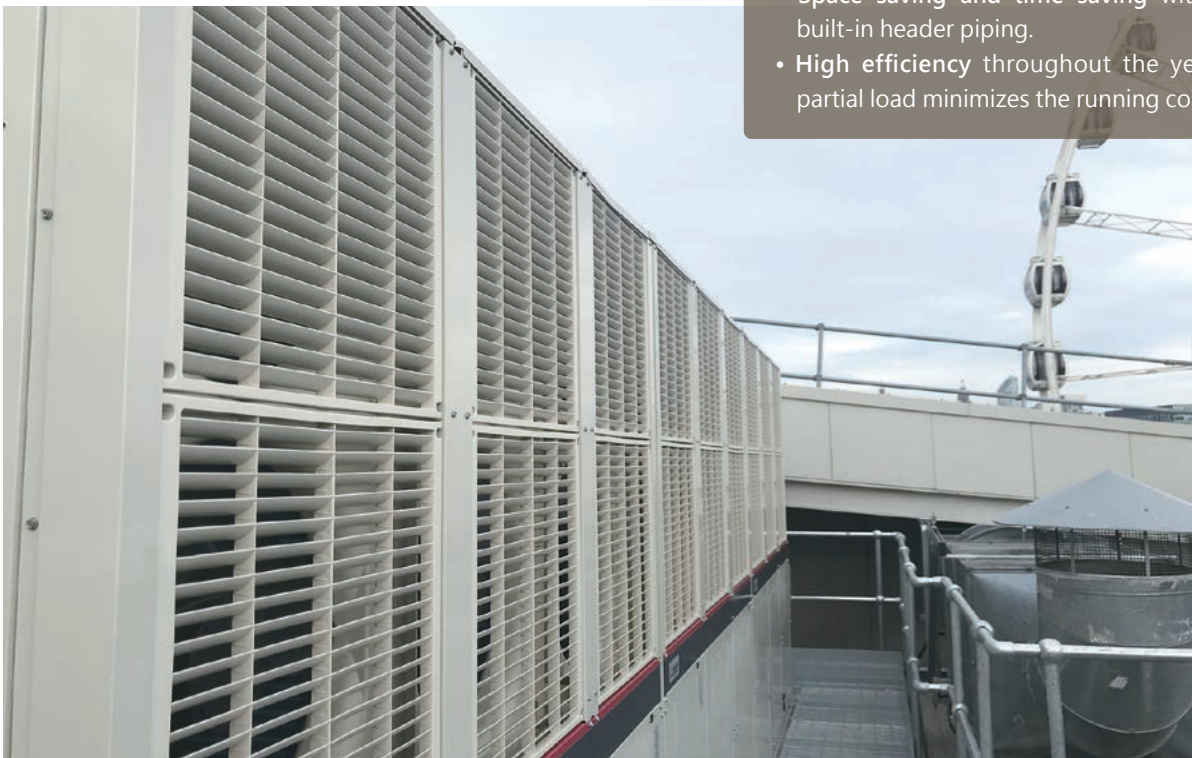
e-series installation on the plant decks
