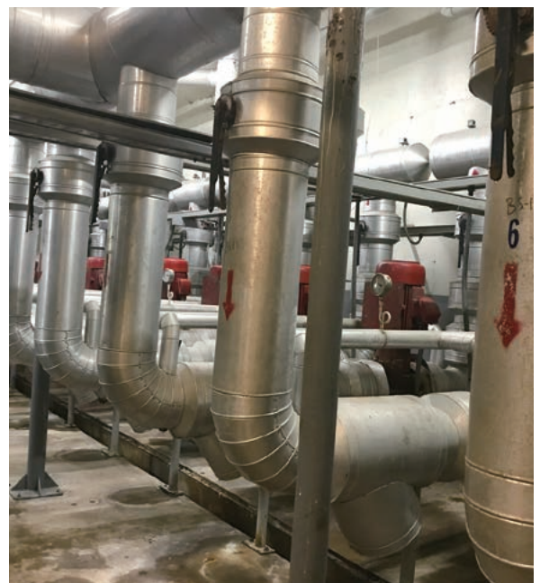
Water pipes and pumps installed in the mechanical room located below the unit.
