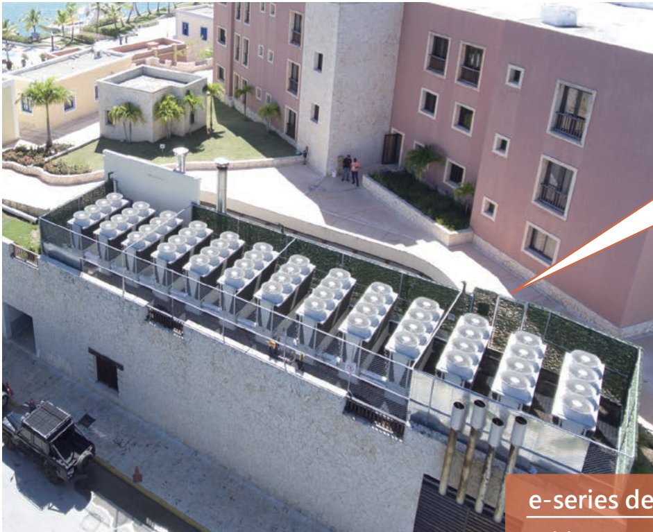
Collective installation behind the building. Originally, the space was occupied by the cooling tower of the water-cooled chillers.
