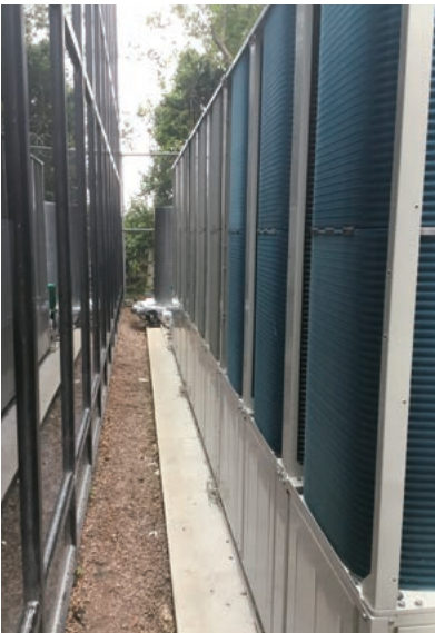
Single-row installation of the e-series along the building
