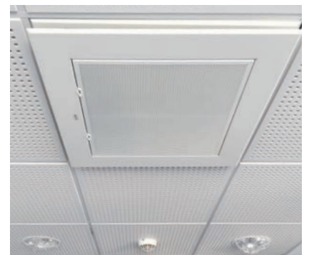
Total of 175 fan coils connected to the e-series
